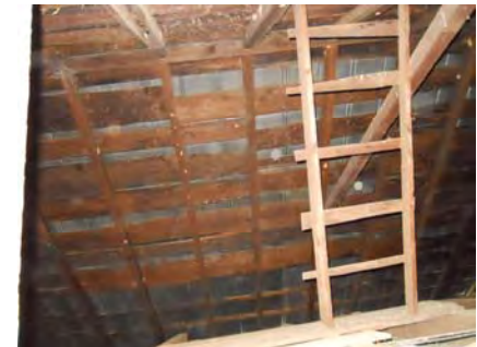
Figure 21 The roof is framed with heart pine rafters and thinly sliced wide boards.
