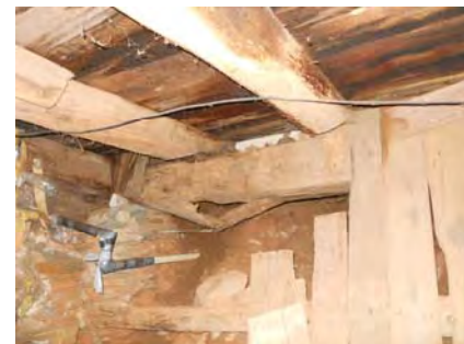
Figure 24 The failing beam under the main floor
