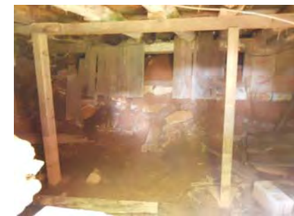
Figure 25 Moisture in the basement
