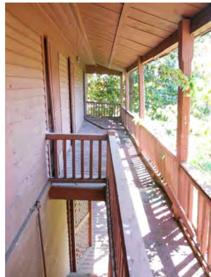
Figure 9 Rear porch - Not accessible
