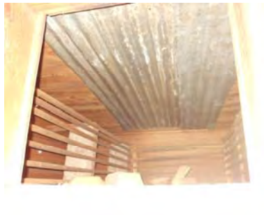
Figure 13 Ice storage area above cold storage
