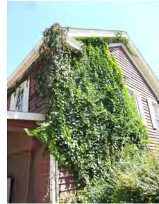
Figure 26 Vines growing on the building should be removed and the building protected from further damage
