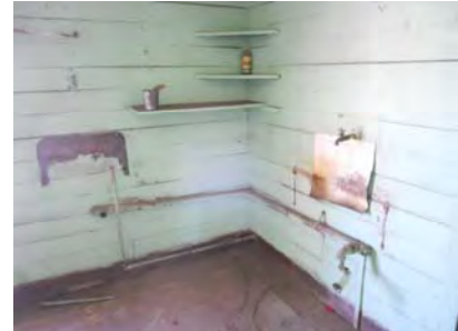
Figure 11 Remnants of a kitchen and plumbing at rear of structure
