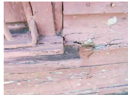
Figure 27 Rotten wood at the joint between the sill and the siding
